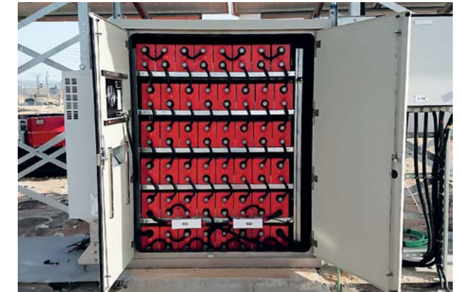
Cooled battery shelter.
