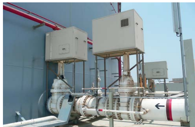
FIRE SHELTERS protecting emergency shut-down valve actuators.
