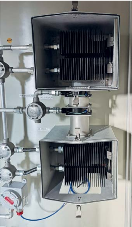
Redundant ventilation fans with pre-warming system.
