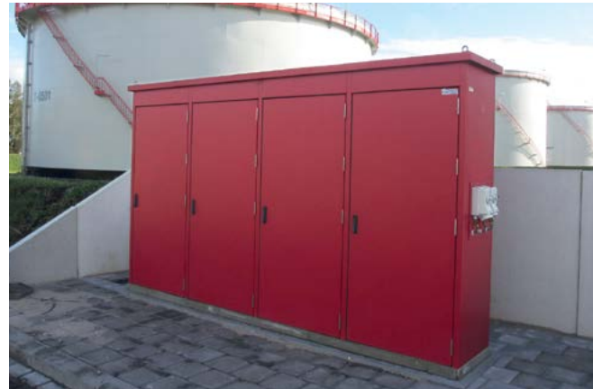
Fire fighting equipment.
