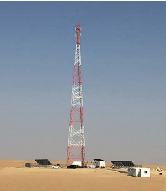
Remote radio station.
