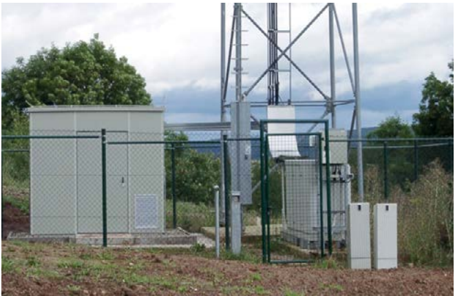
Cellular phone station.
