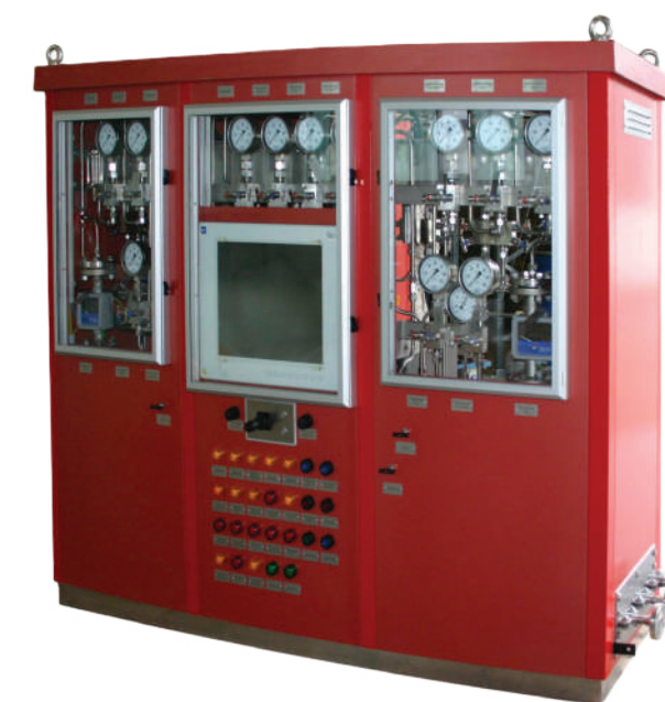
Firefighting Systems Control Panel
